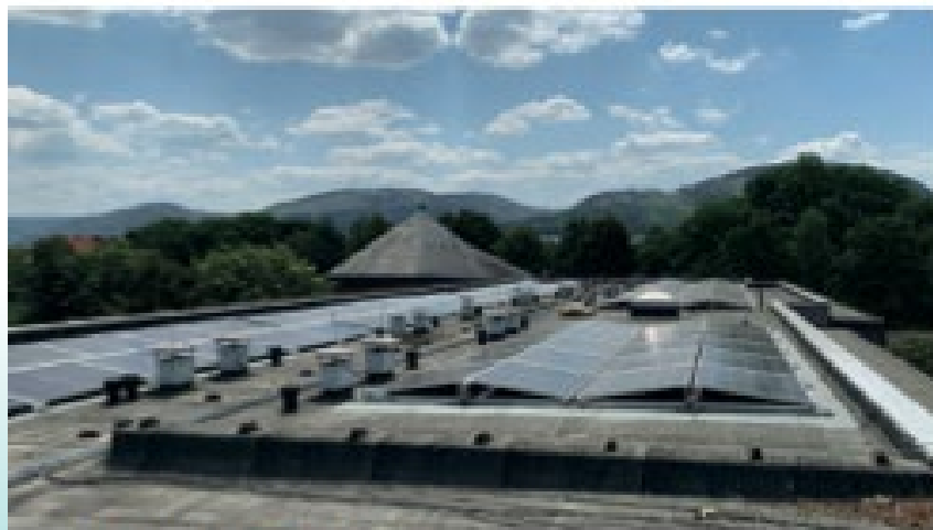
Plaza-Inn Hotel Goslar 114 kWp, 2024
